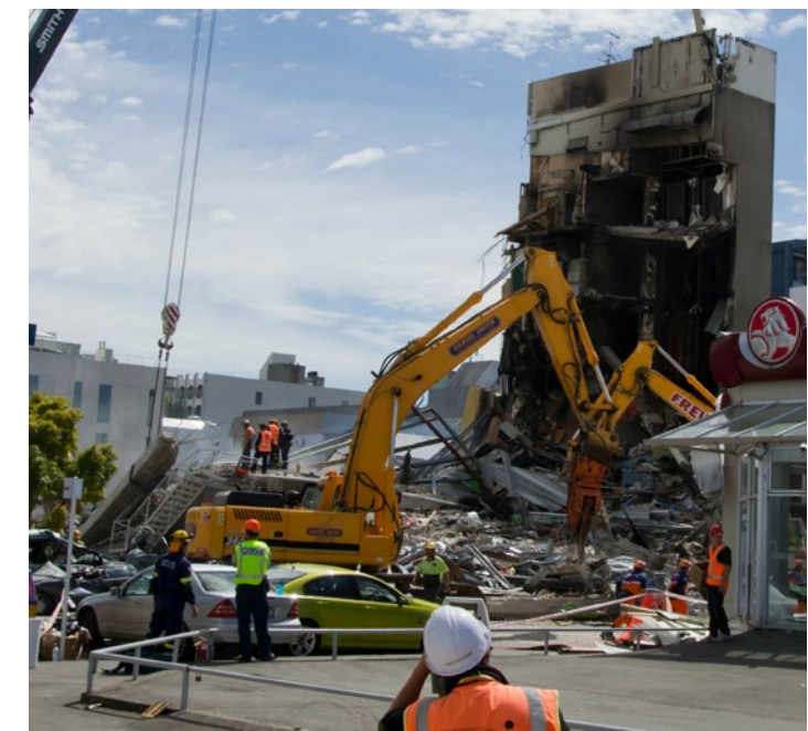
Ruins of the Canterbury Television (CTV) building, 2011 earthquake in Christchurch, NZ. (Source: Wikipedia)
