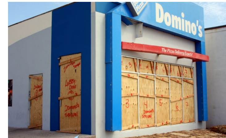
A pizza delivery establishment in Galveston, TX, implemented mitigation measures to lessen the impact of Hurricane Ike in 2008 on their facility. (Source: Robert Kaufmann/FEMA)
